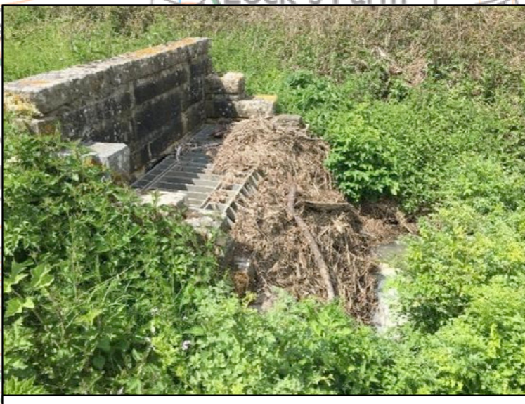
Heavily fouled coarse screening on the downstream entrance to the A283 road culvert at Washington, West Sussex immediately upstream of the proposed crossing site STRX-02
