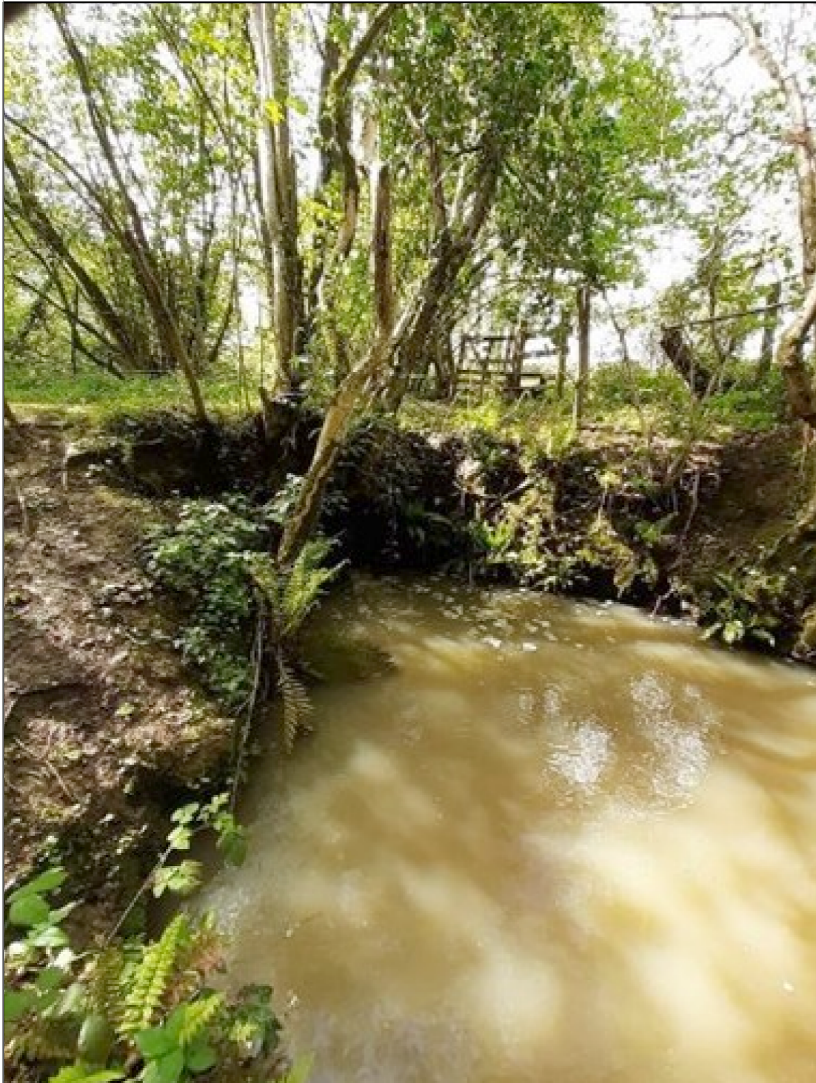
Perched culvert Guessgate Farm stream
