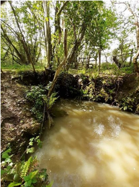
Graphic 4-27 Perched culvert Guessgate Farm stream
