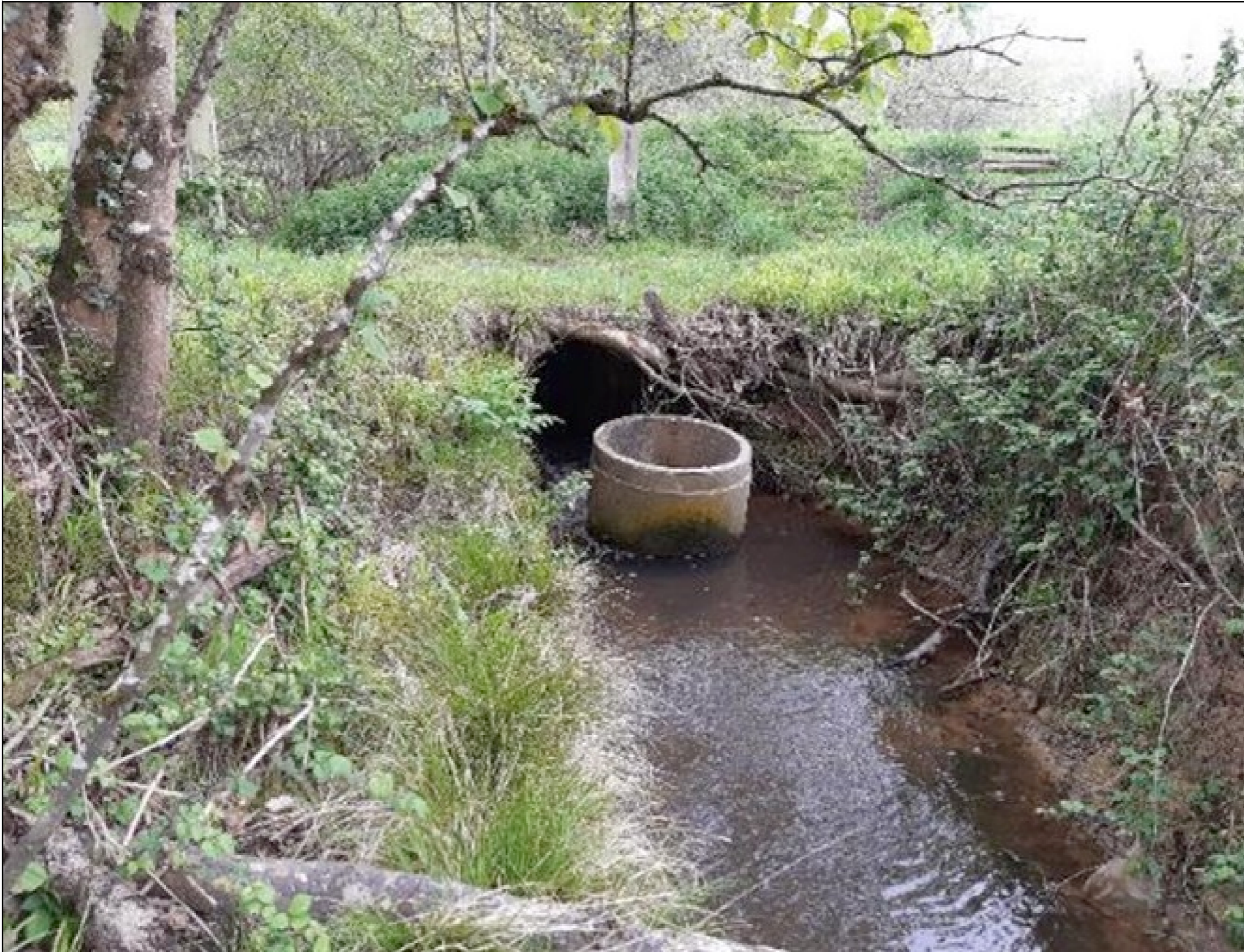
Perched culvert STRX-09
