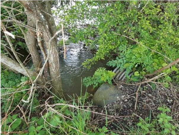
Graphic 4-54 Twin pipes at inlet to downstream lake
